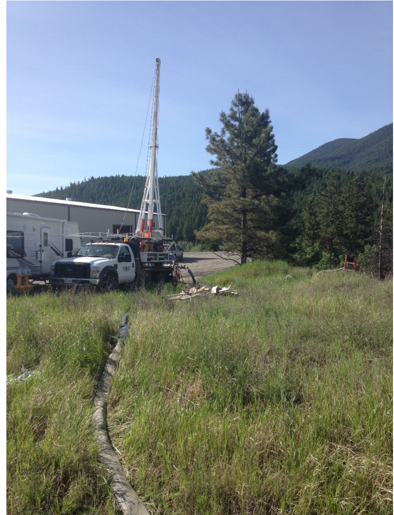
Photo 3 – Well 41015 – Facing South
